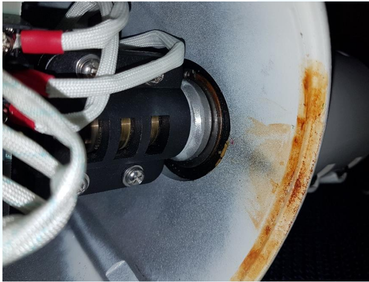
Photo 2 – Water infiltration – Customer photo
